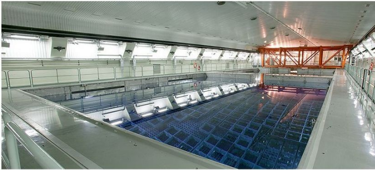
Water-filled storage pools at the Central Interim Storage Facility for Spent Nuclear Fuel (CLAB) facility in Sweden. Storage ponds at reactors, and those at centralised facilities such as CLAB in Sweden, are 7-12 metres deep to allow for several metres of water over the used fuel (assembled in racks typically about 4 metres long and standing on end). The multiple racks are made of metal with neutron absorbers incorporated. The circulating water both shields and cools the fuel. These pools are robust constructions made of thick reinforced concrete with steel liners. Ponds at reactors are often designed to hold all the used fuel produced over the planned operating lifetime of the reactor.
